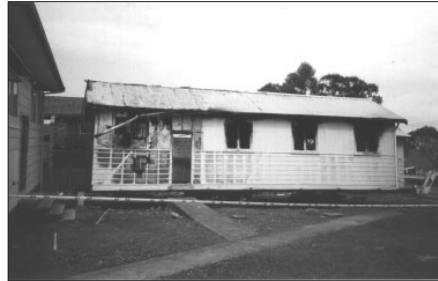
St David's, Toukley, gutted after an arson attack.
